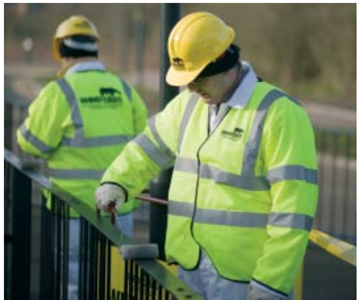
Our large, ongoing project with Coventry City Council involves applying specialist coatings to guard railings, lamp columns and hundreds of items of street furniture.
